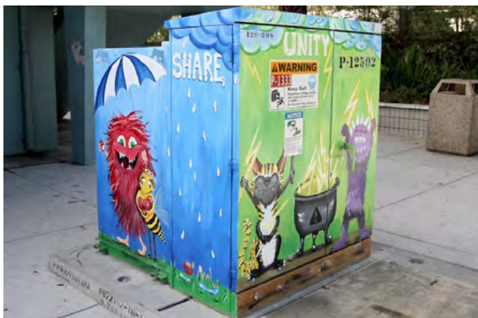
Utility equipment unable to be screened has been enhanced through an art mural.
