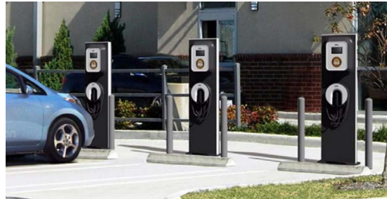
EV Charging Stations
