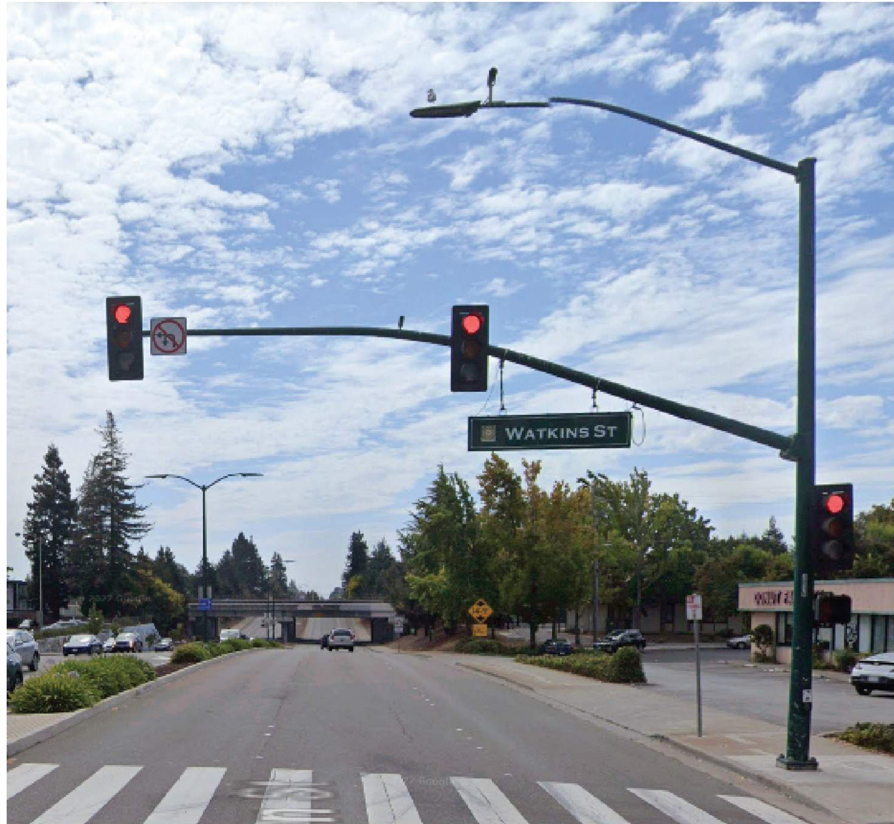
CITY OF HAYWARD TRAFFIC SIGNAL & STREET LIGHTING
