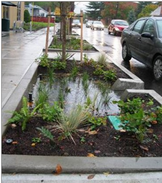
A bioretention area with gutter modification to allow inflow of stormwater.
