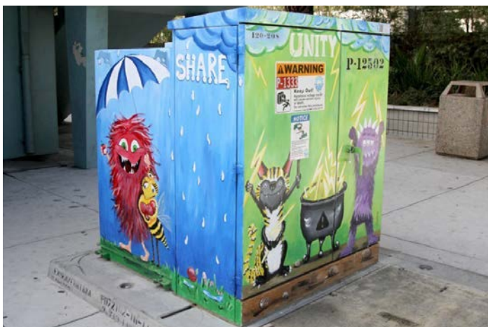
Utility equipment unable to be screened has been enhanced through an art mural.
