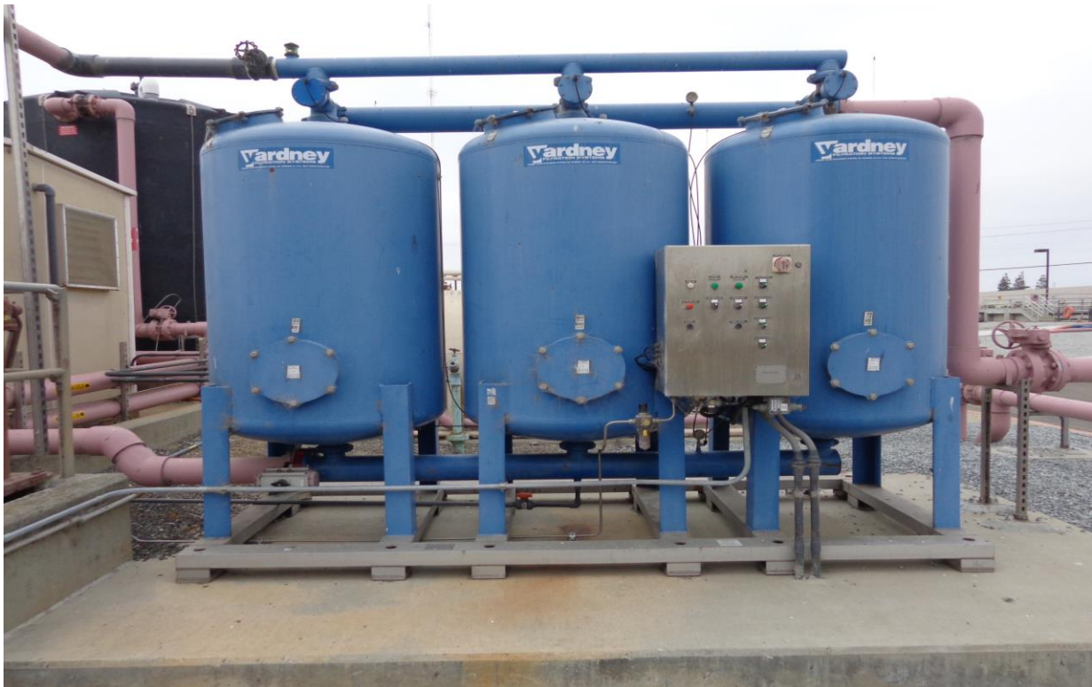
Existing Reclaimed Water Pressure Filters
