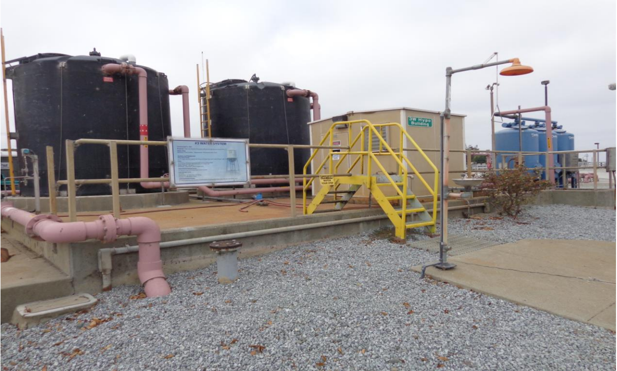
Existing Plant Reclaimed Water System
