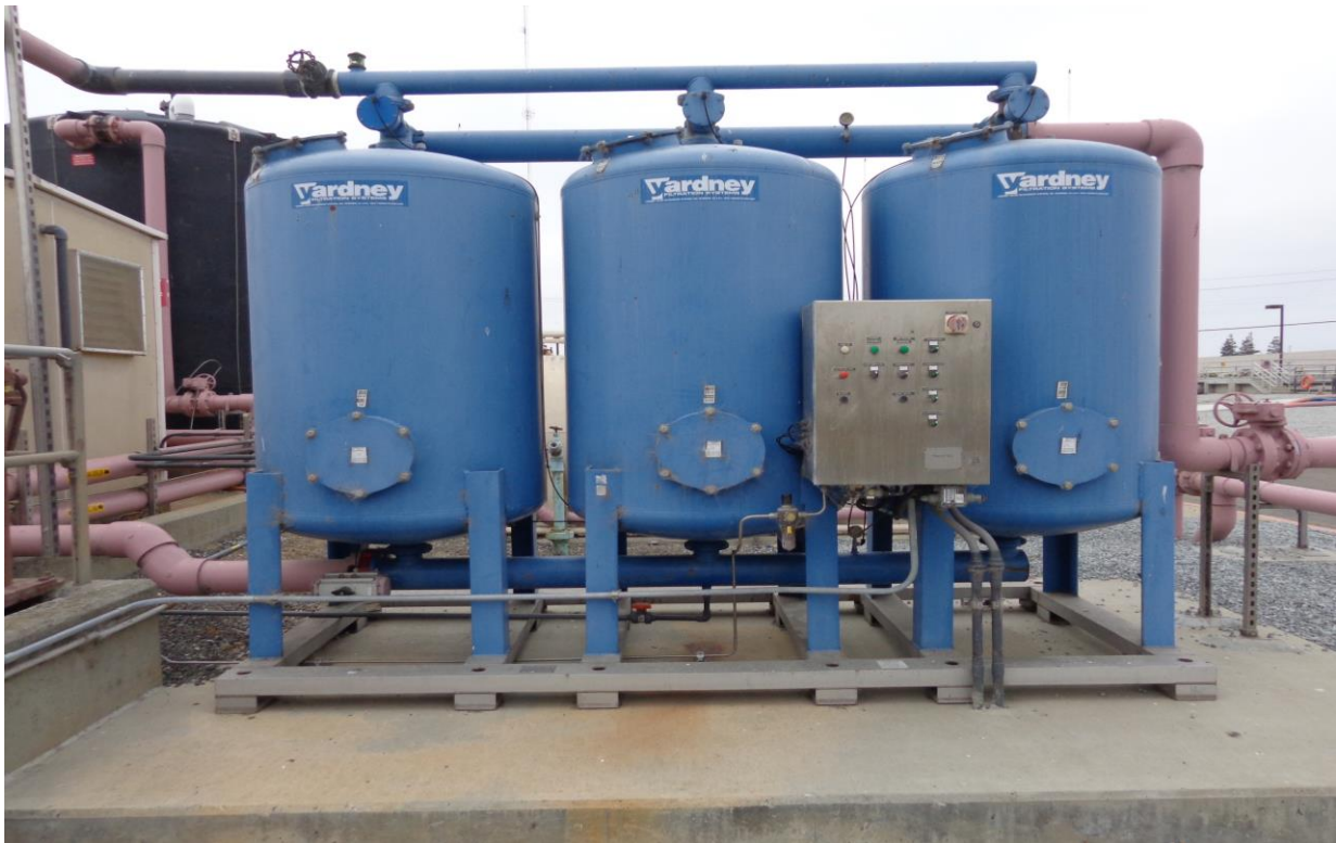
Existing Reclaimed Water Pressure Filters
