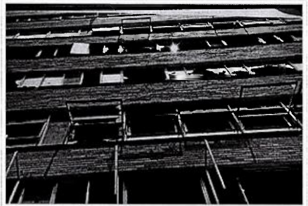
An observer could see straight through the buildings of Pruitt-Igoe due to the large number of broken windows.
