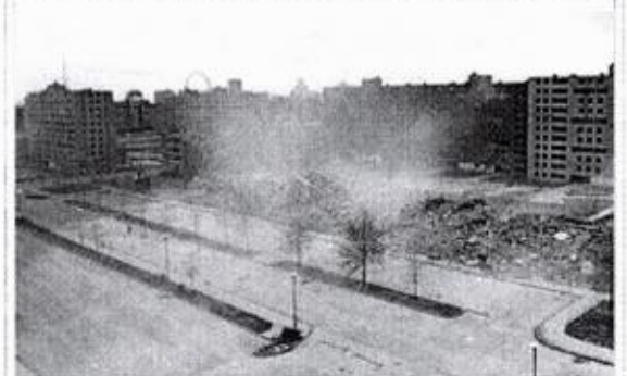
April 1972. The second, widely televised demolition of a Pruitt–Igoe building that followed the March 16 demolition. [1]
